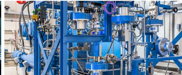
Gas Testing Laboratory
